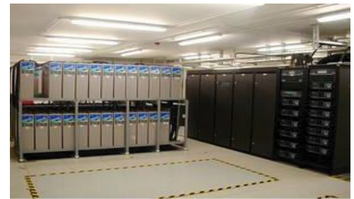
DC Plant Area
